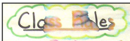
Mrs. Campbell's 4 th grade "Class Rules" sign suffers the effects of water drops through a leaky roof. No more leakiness after Saturday!
